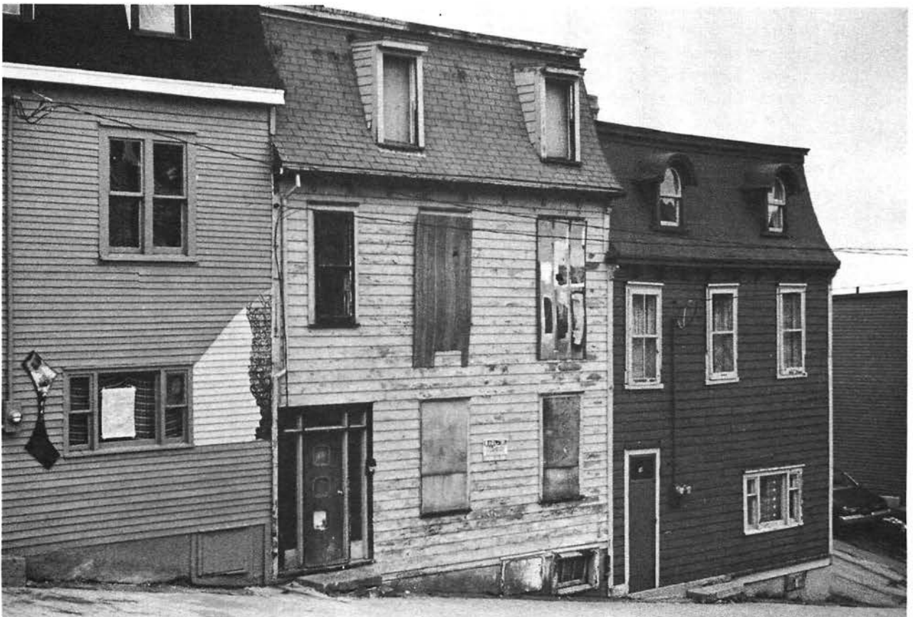
A dilapidated, vacant house on Victoria Street.
