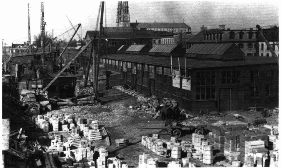
Figure 11 The stone cutting shop on Sussex Drive, fall, 1916. Three derricks used to move the stone were located in the adjacent yard. This site is now occupied by the recently completed (2000) American Embassy. Notre Dame Basilica can be seen in the background. Samuel J. Jarvis collection, National Archives of Canada PA 24996.
