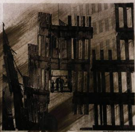
The Final Pieces Welders attached cables to the remaining facade of 2 World Trade Center yesterday in an unsuccessful effort to pull it down. What is left of the building is scheduled to be demolished today.
