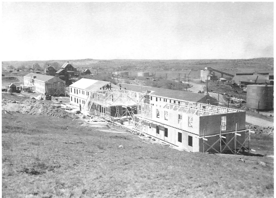
Wartime Housing Limited "Staff Houses" under construction in north end Halifax, 1941. Staff houses were barracks-like structures built to house single male workers. Although not intended to outlast the war, they served as "emergency shelter" housing well into the 1950s. Some were converted into apartments and used by Dalhousie University as married students' residences. (SOURCE: Public Archives of Nova Scotia, Bollinger Collection #11)
