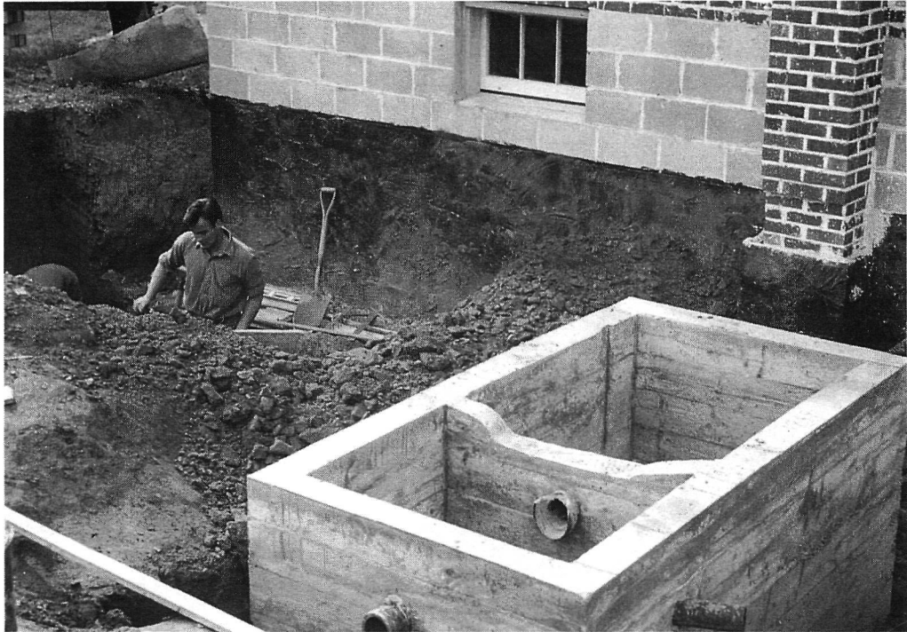
Figure 14: The septic tank was poured, and Harry Hall prepared to frame in the cistern, September 1949.
