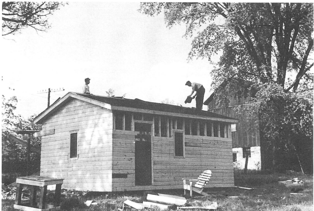
Figure 2: Bill Cameron (left) and Harry Hall (right) building the cottage that the Hall family occupied during the construction of their VLA home, May 1949.
