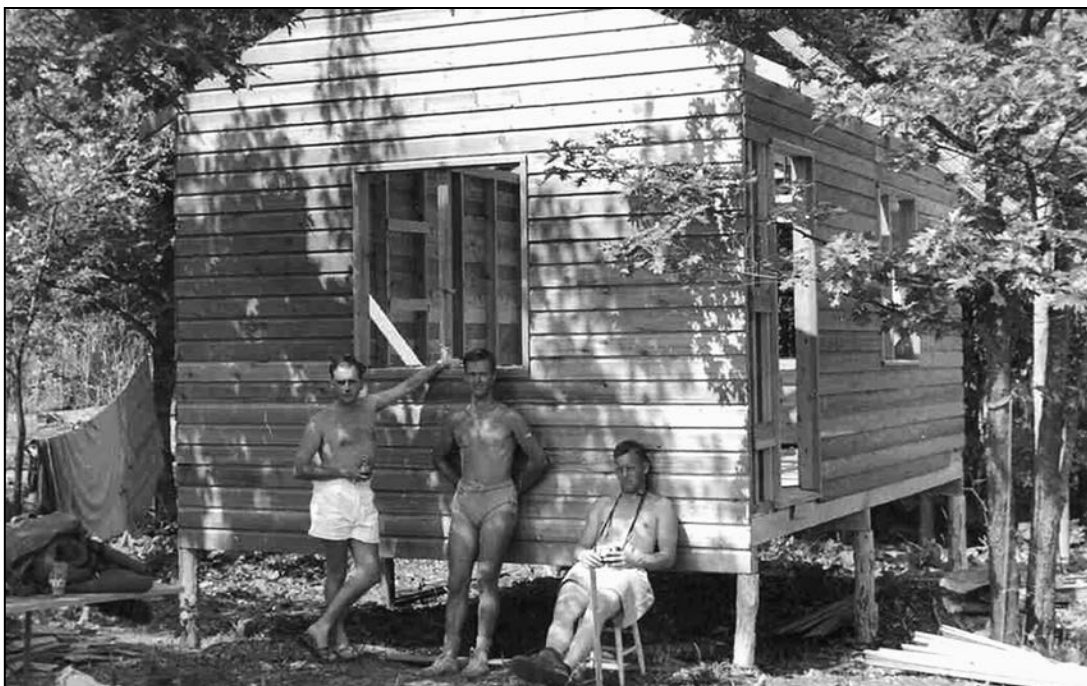
Three men take a break while building a simple cottage at Sixmile Lake, 1953. The postwar boom made cottage ownership possible for a wider portion of the general population. Photo courtesy of G. Crombie.
