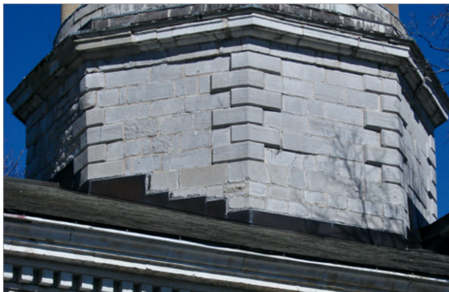
FIG. 16. ST. GEORGE'S ANGLICAN CHURCH, OCTAGONAL BASE OF TOWER, 1841-1842. | PHOTO: PAUL CHRISTIANSON, MAY 2022.
