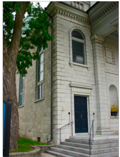
FIG. 38. ST. GEORGE'S CHURCH; DETAIL OF STONEWORK ON RITUAL SOUTH (1839-1841) AND WEST (1842) FAÇADES. | PHOTO: PAUL CHRISTIANSON, MAY 2020.
