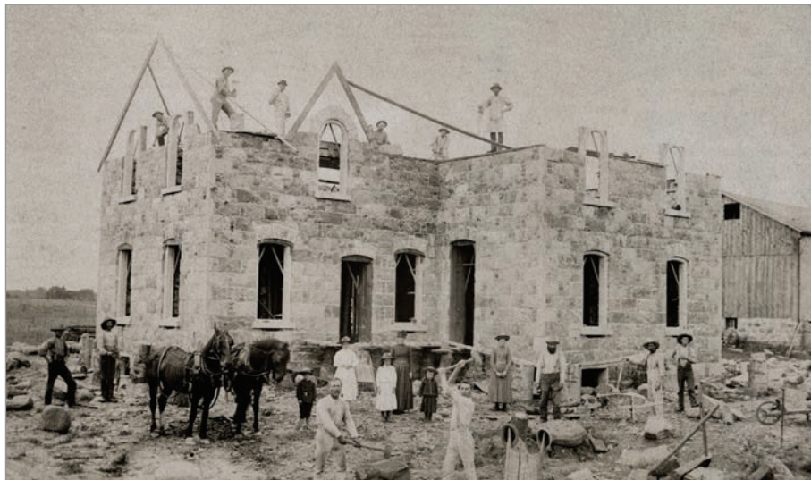
FIG. 22. LAWRENCE HOUSE, CONSTRUCTION SITE, 1891, 205 ALLEN ST., THAMESFORD, OXFORD COUNTY. | AMERICAN AGRICULTURIST , 1894, SPECIAL THANKS TO LISA BICUM AND GEOFF ELLIS.
