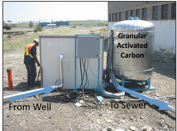
Figure 1. Treatment train for removing cVOCs from groundwater at the site in Case Study #1.
