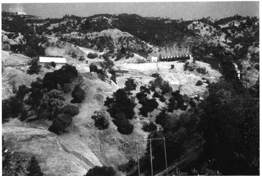
Figure 2 Three of the approximately 20 power units of The Geysers, California, USA, where electrical power is generated from a dry-steam resource.
